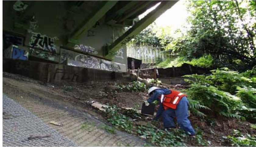
Seattle Department of Transportation already monitors some bridges, such as the Admiral Way Bridge, due to erosion concerns. Photo Source: Seattle Department of Transportation
